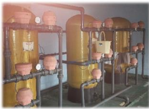
Filters at WTW's
