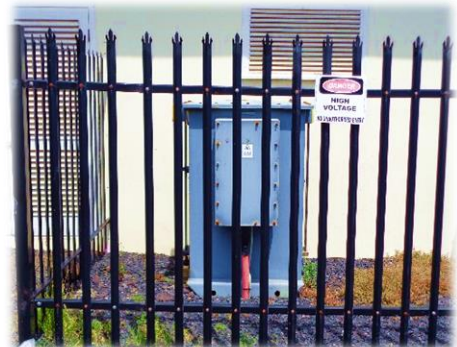
Ground mounted transformer
