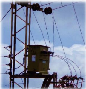
Pole mounted transformer
