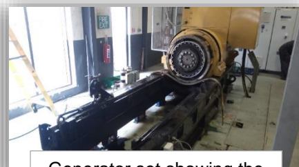
Generator set showing the engine block and sump taken out and alternator still in position
